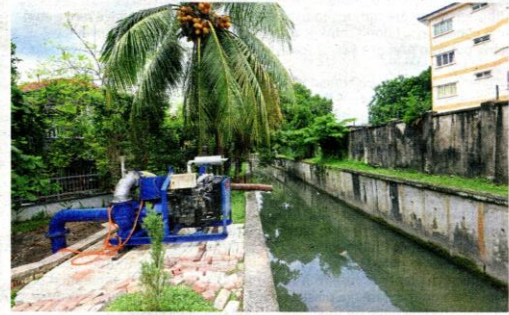
A temporary pump has been installed to direct water into the river should flooding occur. — Photos: ONG SOON HIN/The Star
